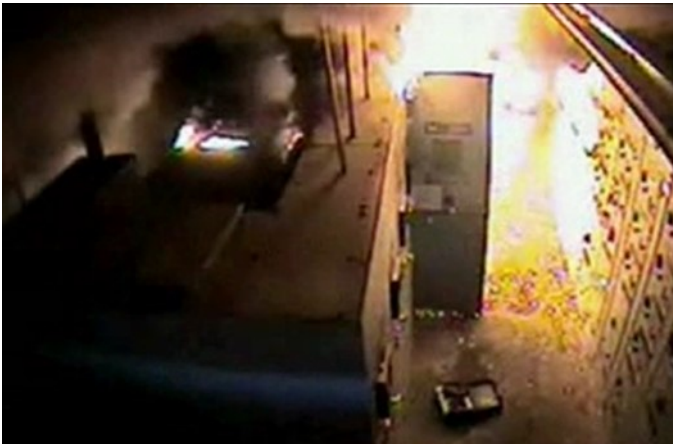
Fig A: Person engulfed in an electrical arc flash during work with open switchgear doors
